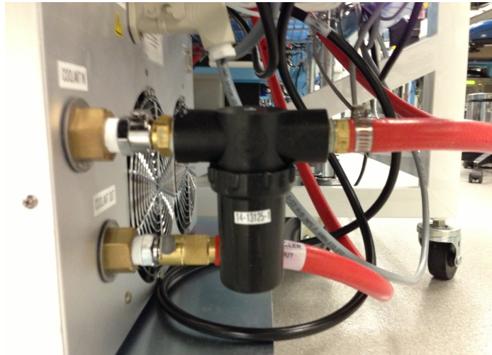
Figure 7-4 Plug hose back into chiller
